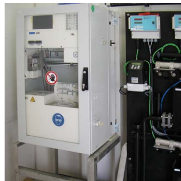
Export project: TOC at a Waste Water Treatment Installation
