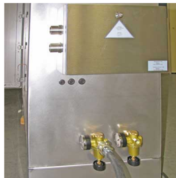
Air inlets for cooling and purging
