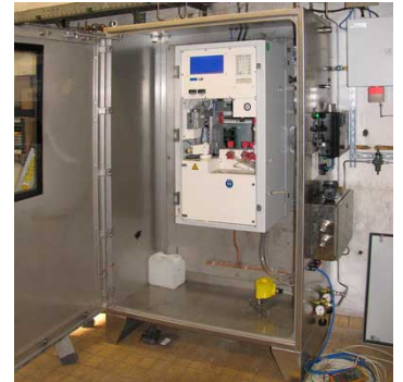
The EEx p cabinet complete with a LAR Quick-COD analyzer
