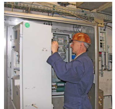
Good access for maintenance is "a must".
