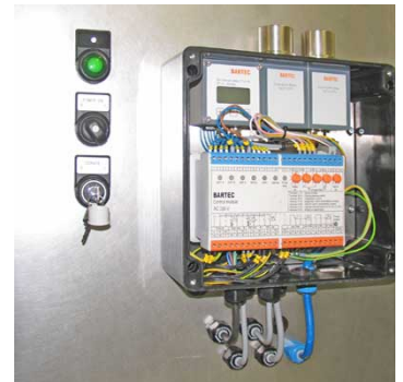
The purge air control unit
