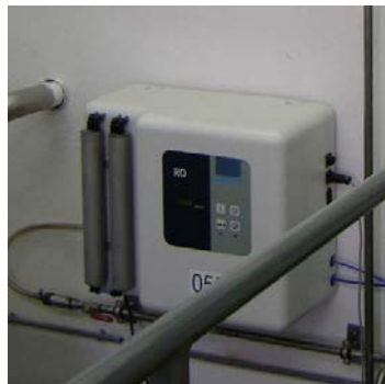
De reverse osmose water unit
