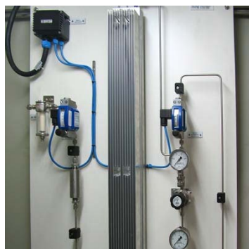
ODS sample conditioning with heat exchanger to air
