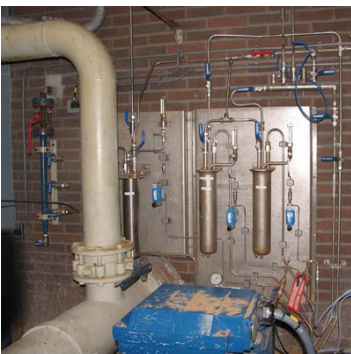
Sample conditioning systems in a boiler house
