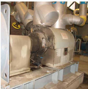
High pressure boiler feed water pump
