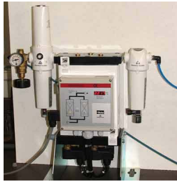
Instrument air is "cleaned" via a maintenance free zero air generator
