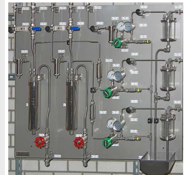
Multi-stream sample conditioning panel
