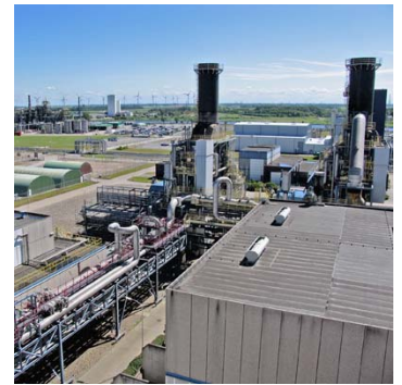
Power plant with co-generators
