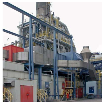
Co-generator; feed water monitored by the Quick-condensate TOC-analyser
