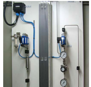
ODS sample conditioning system with a heat exchanger with use of ambient air
