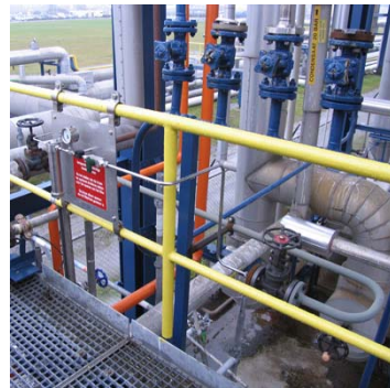
Sample filtration filter panel with primary particle filter, manometer, block valve
