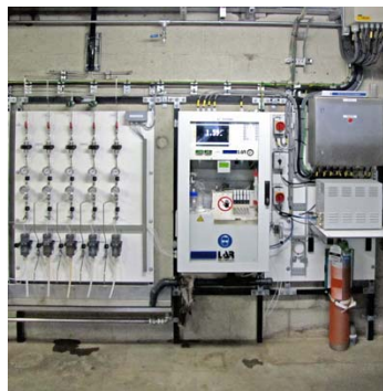
5-stream TC-analyser installation with gas validation
