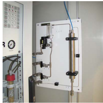
ODS designs and supplies custom made sample conditioning system
