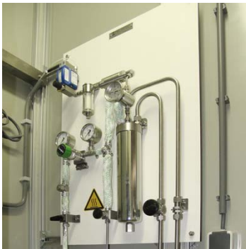
ODS sample conditioning system with a heat exchanger via tap water supply
