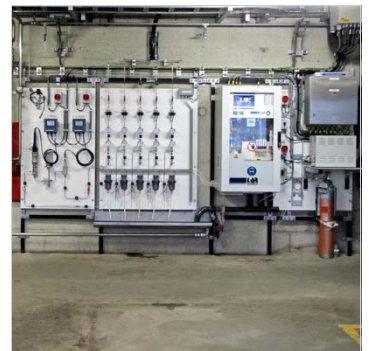
5-stream sample conditioning en TOC-analyser
