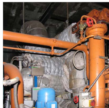
E-generator operates via HP steam.
