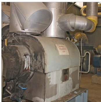
Via a high Pressure Pump for boiler feed water
