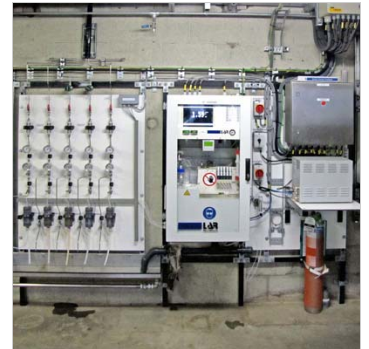
Panel with sample conditioning & multi stream TC-analyser
