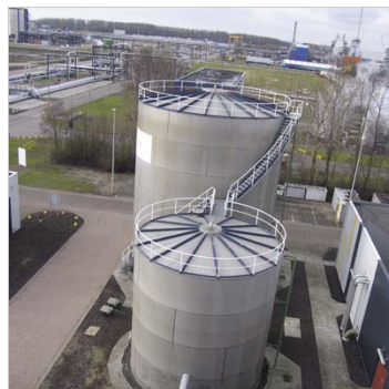
Buffer tanks with boiler feed water
