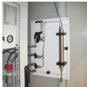
TOC-analyser with sample conditioning panel
