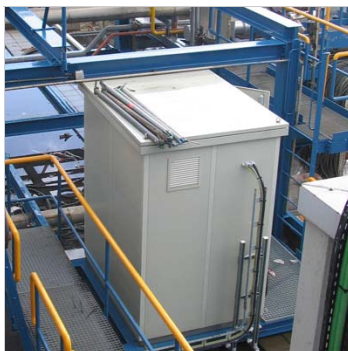
Walk in shelter at a chemical site
