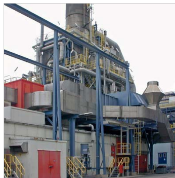
Power plant generates E-power and steam for chemical plants
