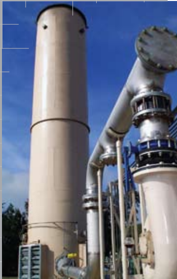
Photo courtesy of LFG Specialties
