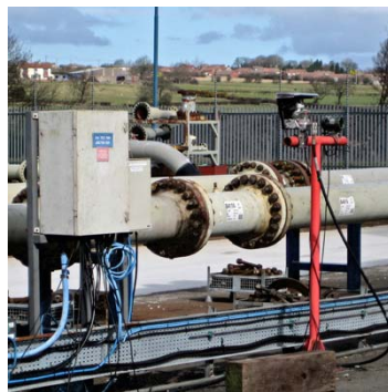
Meter installed at Advantica.
