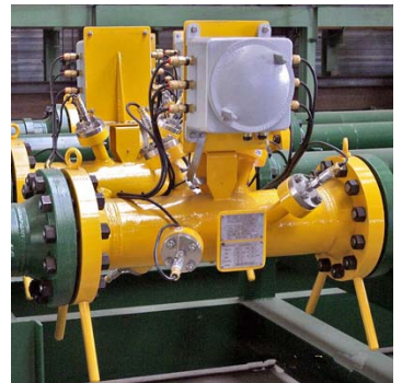
The loading meter is mounted into the meter run.
