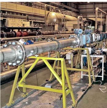
Meter run with multiple beam ultrasonic meter.
